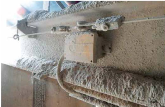
The ambient conditions pose a challenge to electrical and especially safety-critical components.
