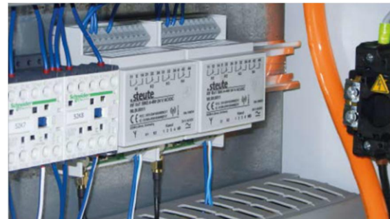
The receivers and evaluation units of the two wireless foot controls are installed inside the control cabinet (image: Carl Geisser AG)
